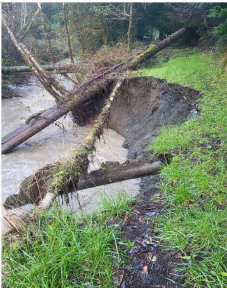
Areas along Indian Creek slide off and into the creek, adding to sediment washing into the fish ladder.
