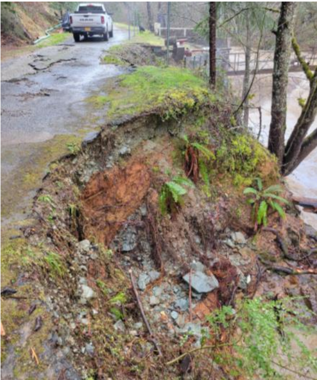
Some outer edges of the entry road are undercut and now have 12' vertical dirt sides.
