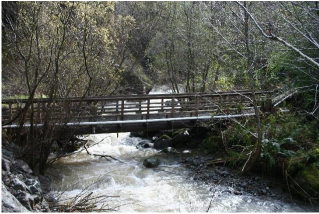
The footbridge to the Indian Creek hatch house was washed away due to the creek flooding.
