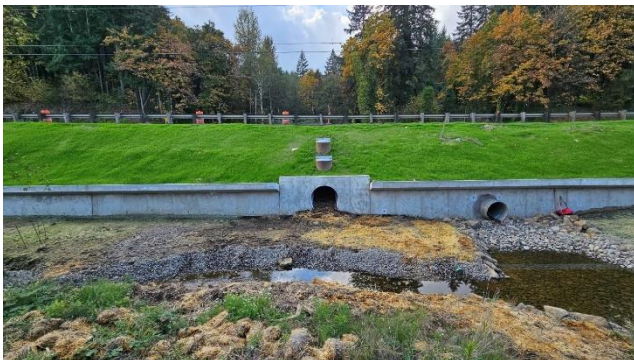
Palensky Wildlife Crossing under Hwy 30, a busy four-lane highway outside of Portland. Photo by CREST.
