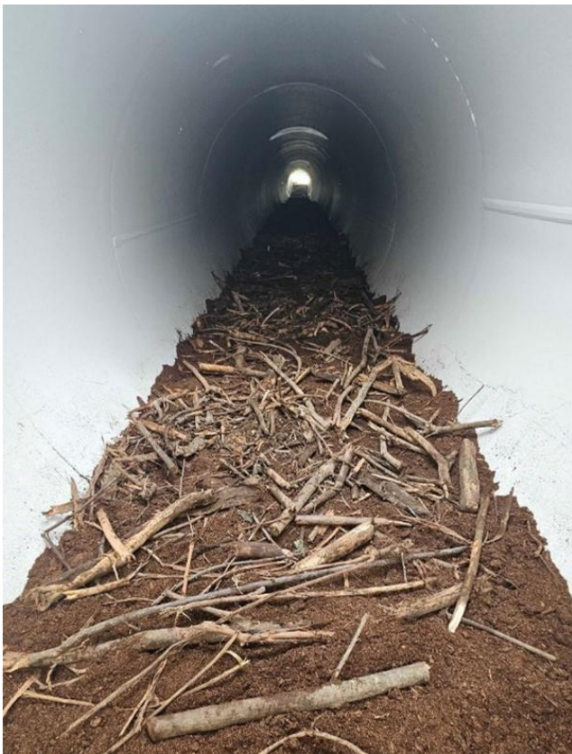
The base of the crossing is covered in several inches of soils, bark, sticks and leaves. Photo by CREST.
